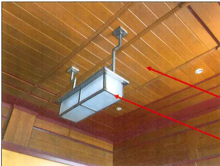
Image 24: Existing ceiling conditions - Added boards where north lobby wall moved and truncated historic light fixture (Waisler, 2016)
