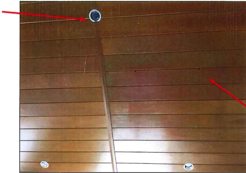
Image 22: Existing ceiling conditions - Recessed 5 inch can lights that cut through wood boards and trim. Holes visible from past ceiling mounted light fixtures (Waisler, 2016)
