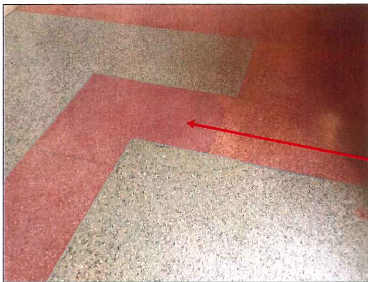
Image 25: Existing floor conditions - Incompatible terrazzo patch (Waisler, 2016)
