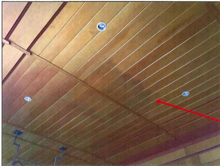
Image 23: Existing ceiling conditions - Staining from past ceiling mounted light fixtures (Waisler, 2016)
