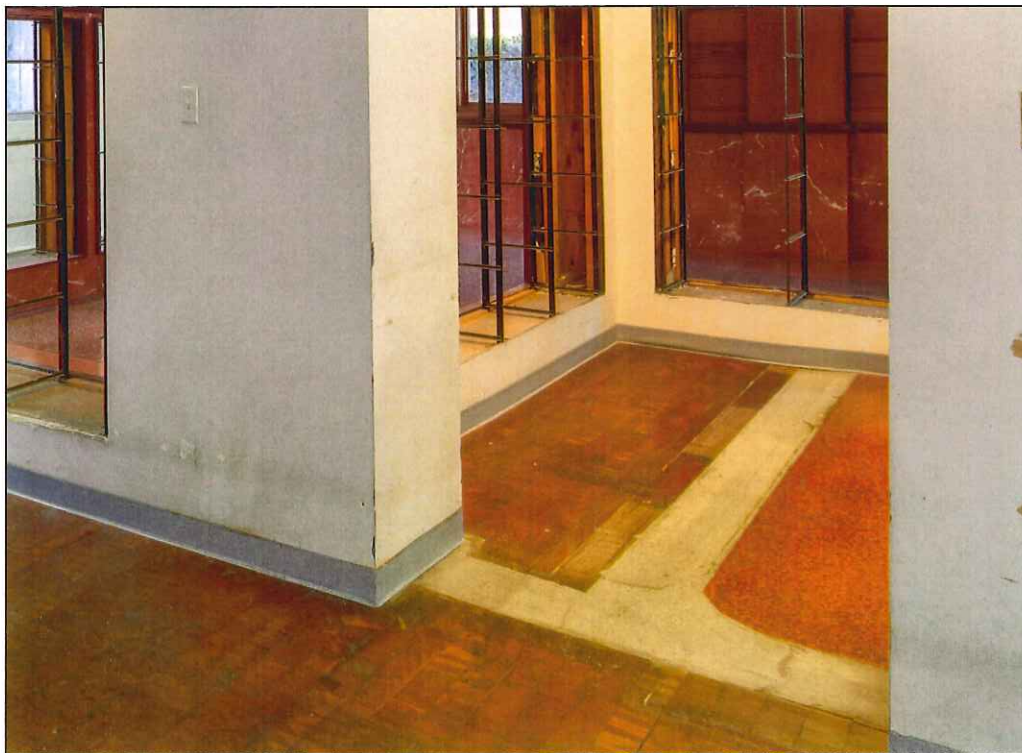
Image 29: View of lobby flooring from inside workroom, looking east. Image shows original location of lobby north wall (where salmon color terrazzo flooring is visible) and north office (where end grain wood block flooring is visible) (Schafer, 2016)
